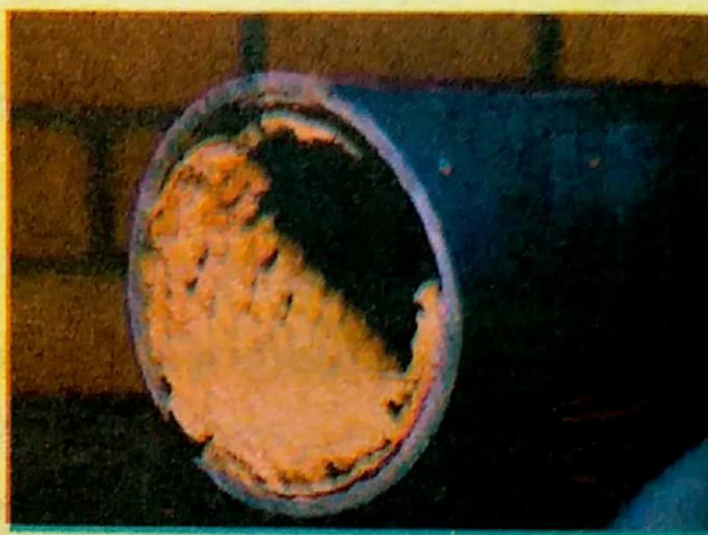
Fig. 15.5: Salts deposition inside of boiler pipes
