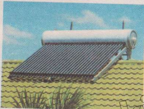
Fig. 5.15 Solar panels installed on the roof
