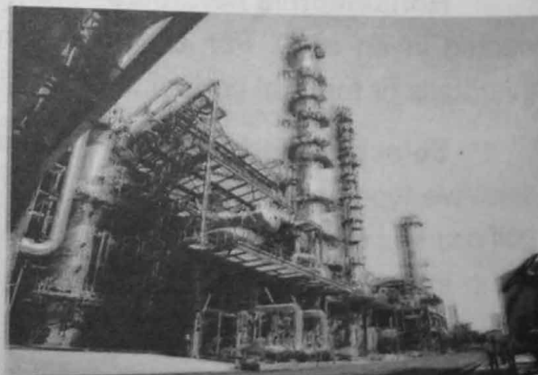
Petrochemical Plant in the Kingdom of Saudi Arabia
